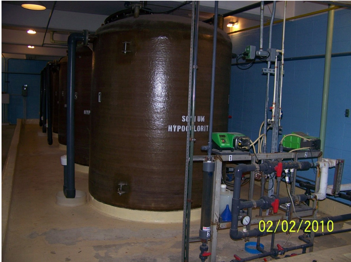
Liquid Sodium Hypochlorite Feed Pumps and Storage Tanks
