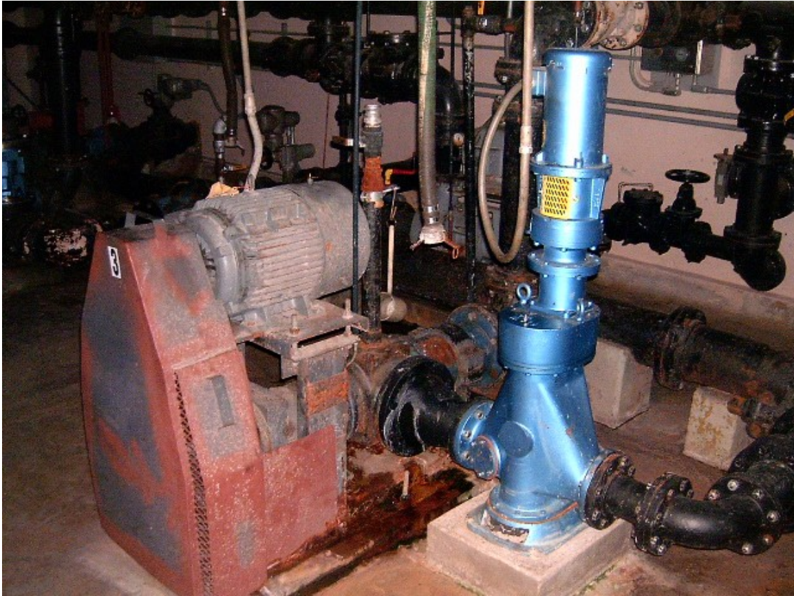
Raw Sludge Pump
